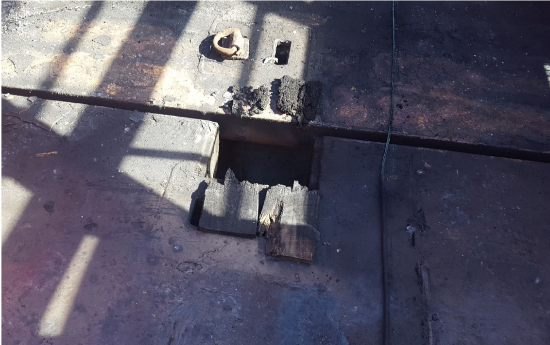
Figure 2: Tween deck gaps
