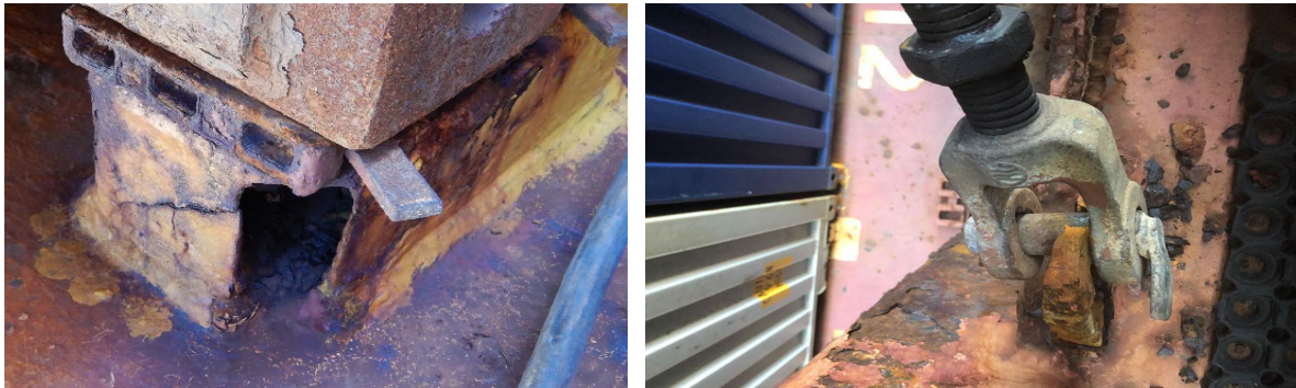
Heavily corroded container securing socket and lashing point
